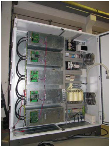
Fig. 9. Switchgear cabinet, with master station (blue) and four slaves (red)
